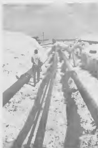
PIPE LEADING out to loading stations will be out of sight when the trenches are filled in. Sleeves, paint and wrapping offer protection from corrosion.
